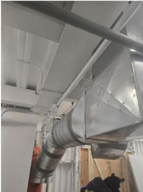
Ducting first floor
