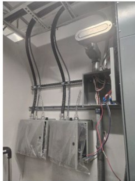
Junction boxes and connections
