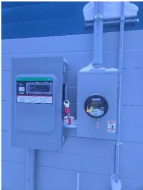
Meter and disconnect
