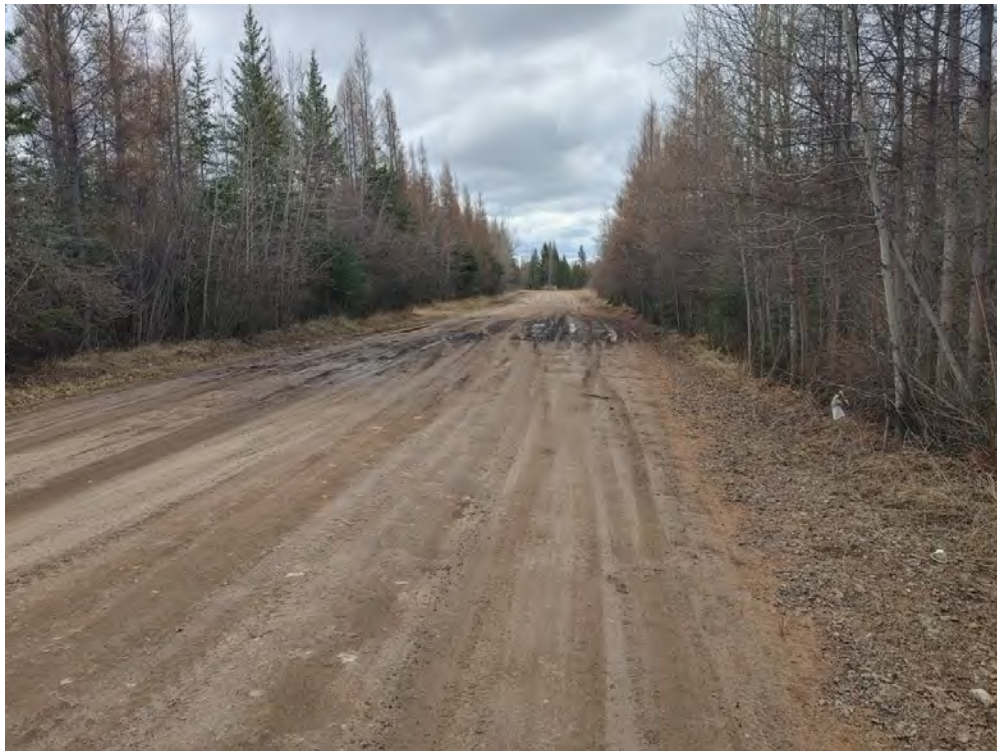
Figure 33: Lagoon Road – May 20
