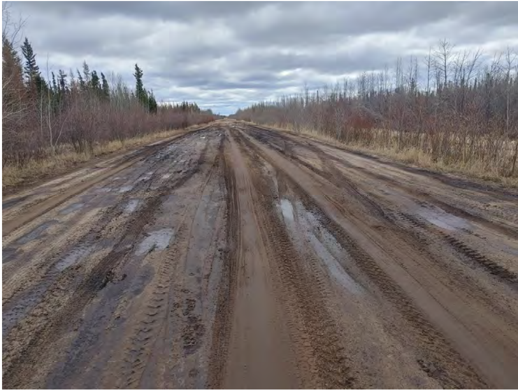
Figure 36: Lagoon Road - May 20
